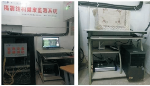
图 6 现场长期采集站 Fig. 6 Located long-time acquisition station
