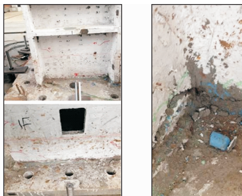
(a) 横墙及纵墙裂缝 (a) Cracks in longitudinal walls and cross walls (b) 首层底部裂缝 (b) Cracks in bottom of the first floor
